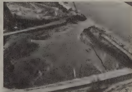
Breaking a dike at on the Puyallup river to help rehabilitate its estuary.
